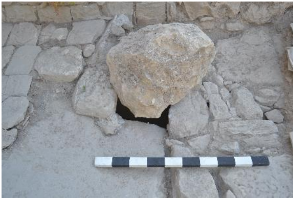
Figure 102: hole in floor above cistern, unsure structural stability, 2016
