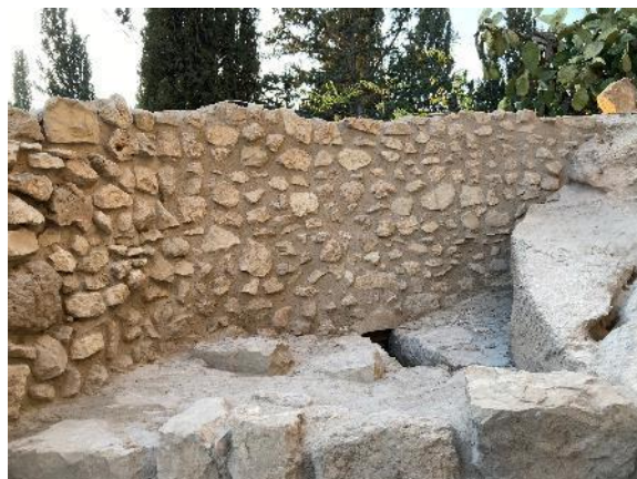
Figure 59: Wall B after measures in 2021: new mortar fillings make the wall stable and prevent new biological colonization; mural crown rebuilt for better water discharge
