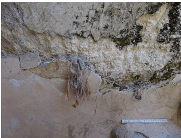
Figure 72: Previous condition of loose and hollow pieces of plaster
