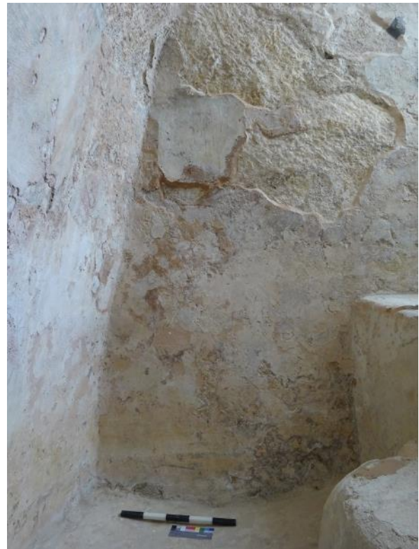
Figure 87: Condition after removal of salt efflorescence and
