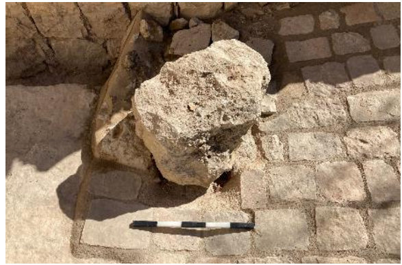
Figure 103: hole in floor above cistern, structural stability ensured after construction measures and retiled floor, 2021
