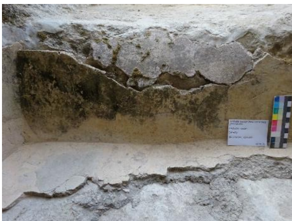
Figure 70: Biological growth on the plaster
