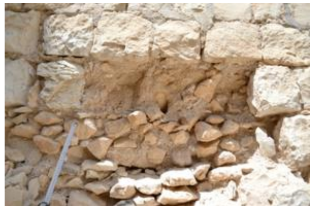
Figure 12: Loss of material wall D (THIERRY, 2017)
