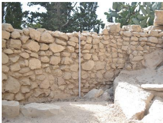
Figure 58: Wall B before measures in 2016: biological colonization, loose mortar and unstable structure, 2016
