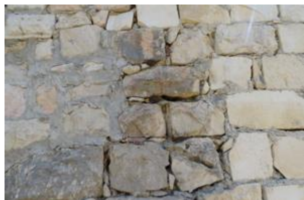
Figure 13: Loss of material in joints (THIERRY, 2017)
