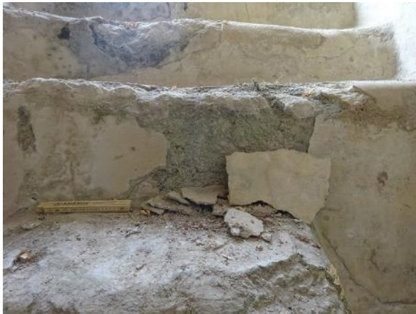
Figure 76: Pieces of plaster which fell off
