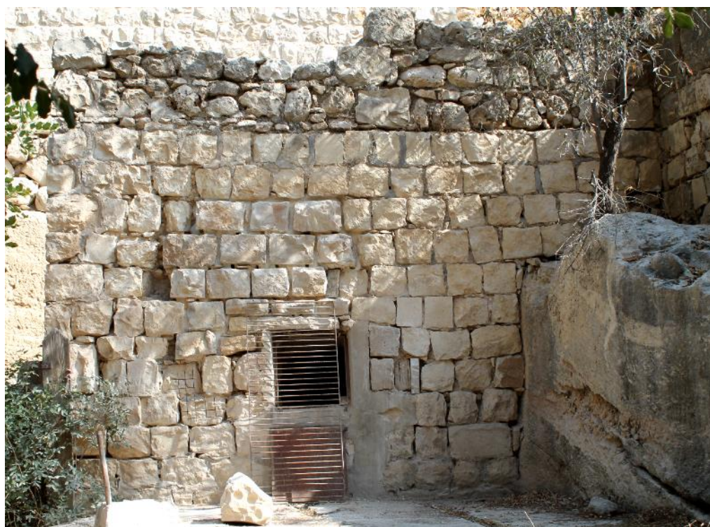
Figure 50: southeastern front of wall D after closing the big missing part, Oct. 2019
