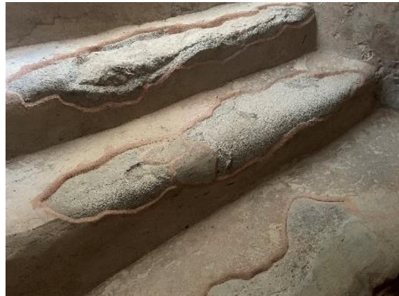
Figure 133: Filled gaps of the 1st century layer by means of a grey repairing mortar and pointing of the orange mortar
