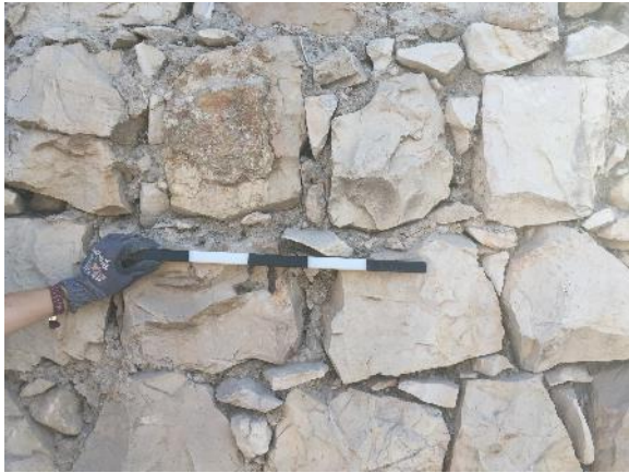
Figure 33: photo documentation area 2: before measure: joint filled with lime mortar, small stones, dirt, loose material, snails and biological colonization
