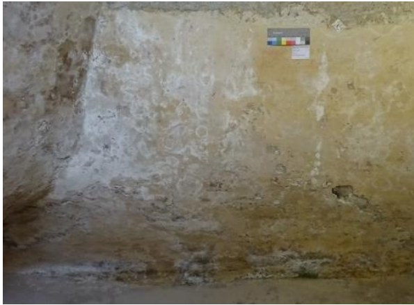
Figure 64: Before removal of salt efflorescence
