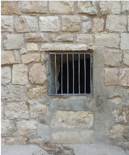
Figure 128: access to cistern in wall D with sustainable long term coverage, 2022
