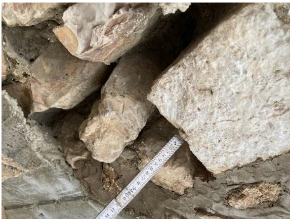
Figure 90: vault after scratching, E. Thierry, 2021
