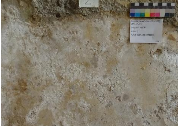
Figure 68: Decay caused by salt before consolidation
