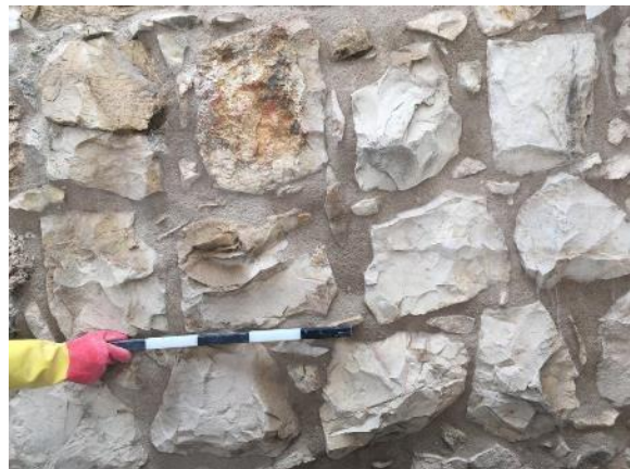
Figure 41: photo documentation area 2: final result: refilling with visible mortar after final smoothing
