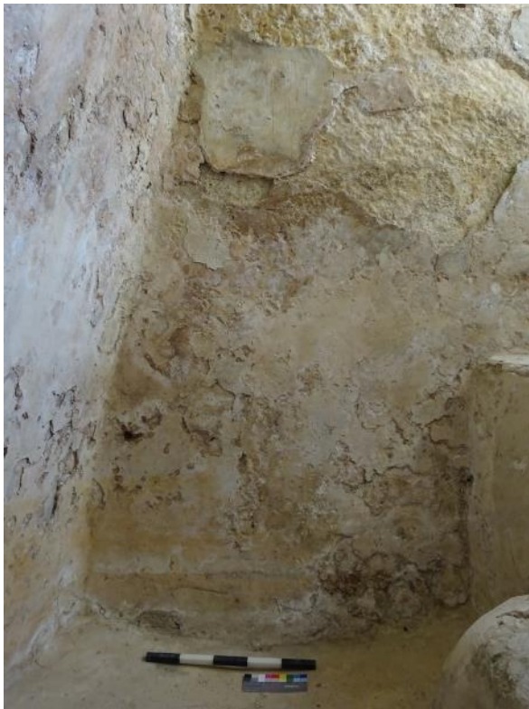
Figure 86: Condition before removal of salt efflorescence and repairing
