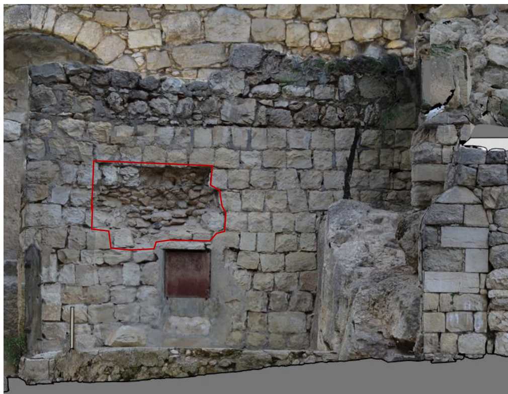
Figure 49 ortho photo, section, view south west on wall D, before measure (big missing part), E. Thierry 2016
