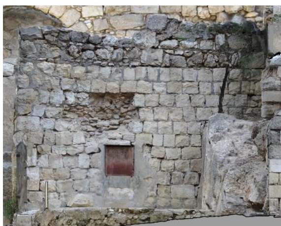
Figure 60: wall D before measures, 2016
