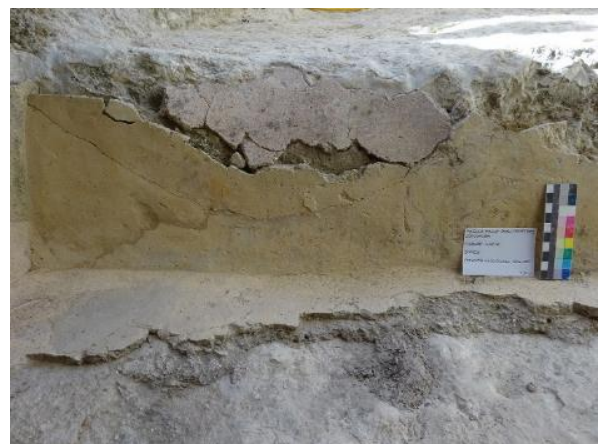
Figure 71: Sample of removed biological growth
