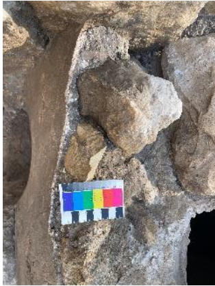
Figure 120: discovered plasters near hole above cistern; bottom plaster: grey lime plaster with chulk, top plaster: fine lime plaster, 2021
