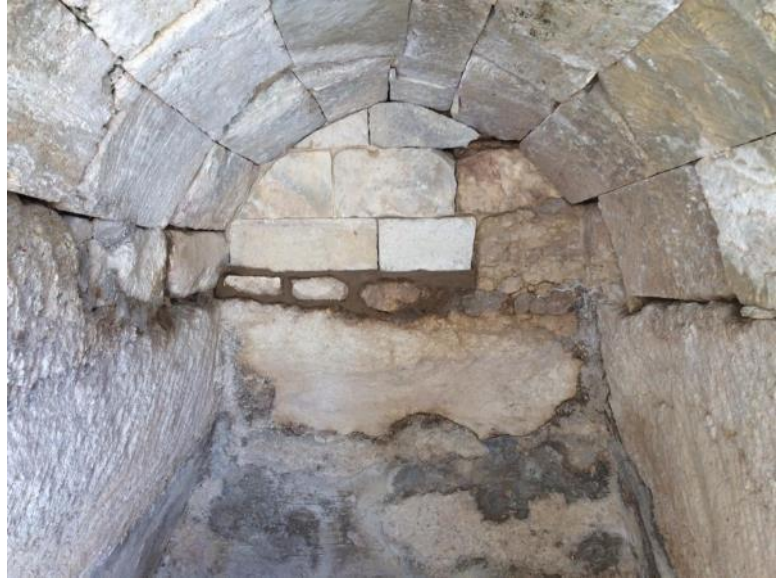
Figure 25: reconstructed vault in original shape, northwestern Miqveh (note: mortar in frontal wall not dried)
