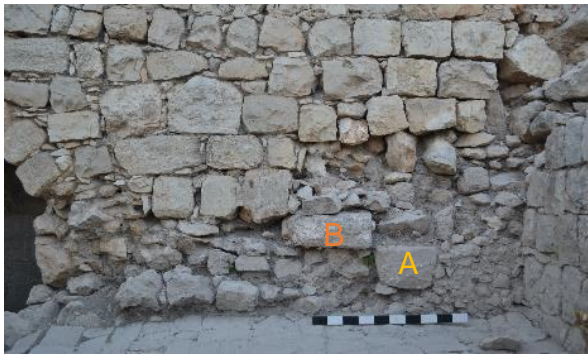
Figure 54: bottom part of big cemetery wall before measures in 2016
