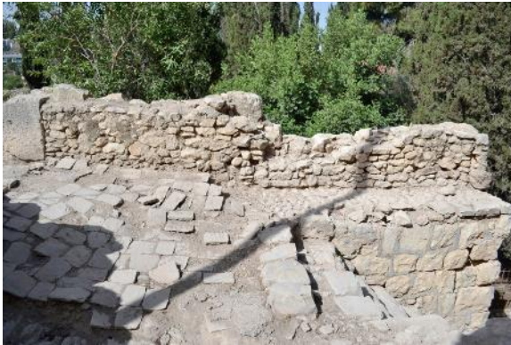
Figure 100: floor and wall C on Miqvot level before measures, 2016
