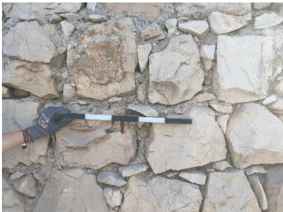
Figure 40: photo documentation area 2: before measure: joint filled with lime mortar, small stones, dirt, loose material, snails and biological colonization
