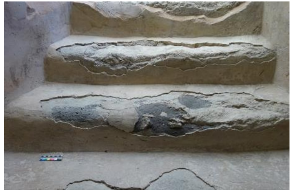
Figure 89: Condition of the stairs after the removal of
